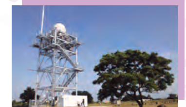
PANDA tower and container installed at the Advanced ICT Research Institute
