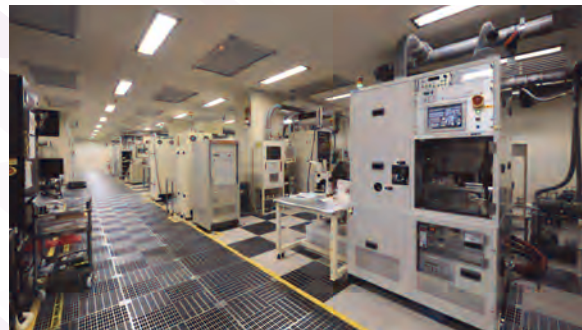
Processing equipments in the clean room
