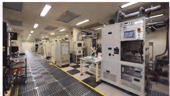
Processing equipments in the clean room
