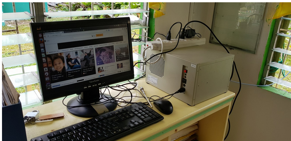
Figure 25. Showing connectivity between AP (Bgy. Hall) and STA1 (Principal's Office)
